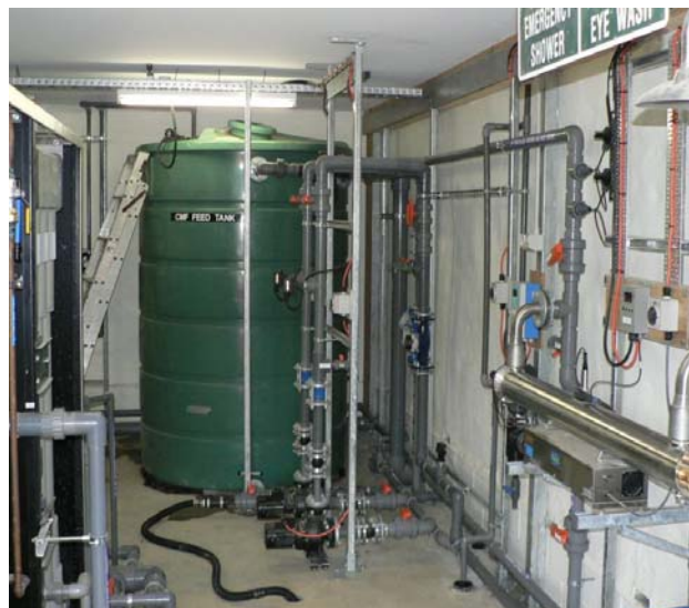
A small waste water treatment plant at the Currumbin Ecovillage allows all waste water produced on site to be treated and re-used on site.
